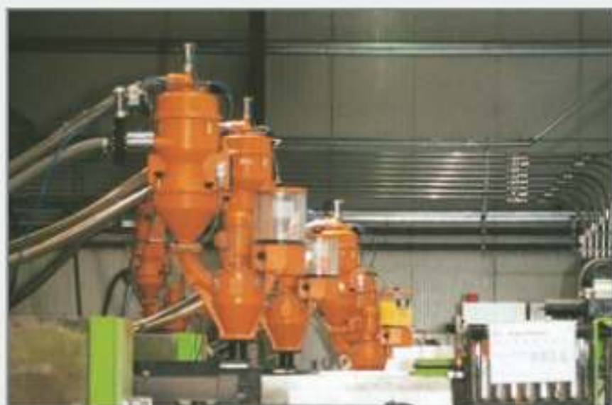
Conveying system with pre-mixers
