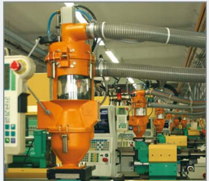
A 2 hopper loader and intermediate hopper Z I in a conveying system
